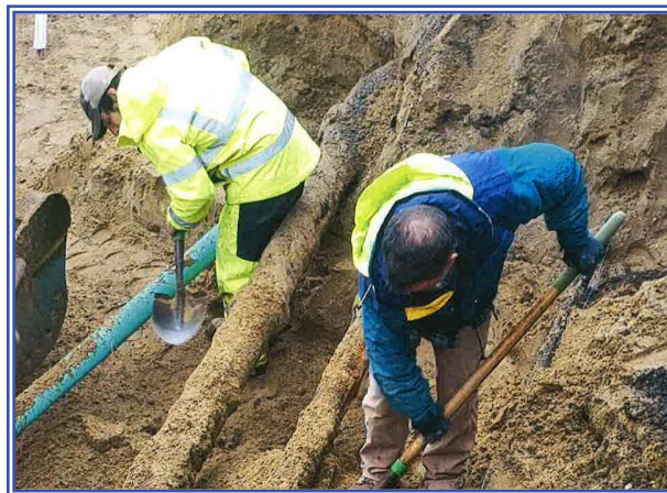
Fire Service Installation
